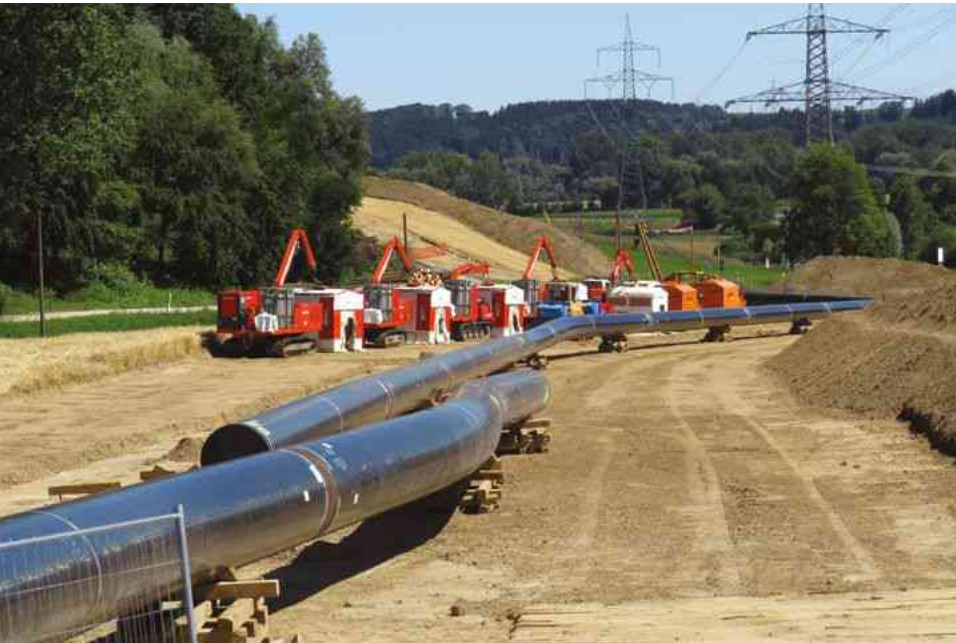
9. Europe has 200,000 km of gas transmission pipelines which could be used for hydrogen transportation. Photo: Vuxi.
