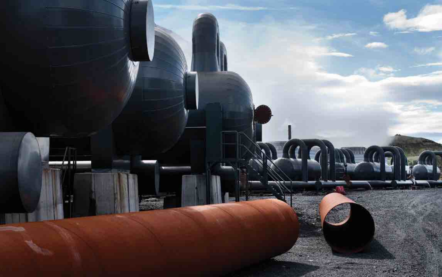
▲ Hengill View of Hellisheidi Geothermal plant.
