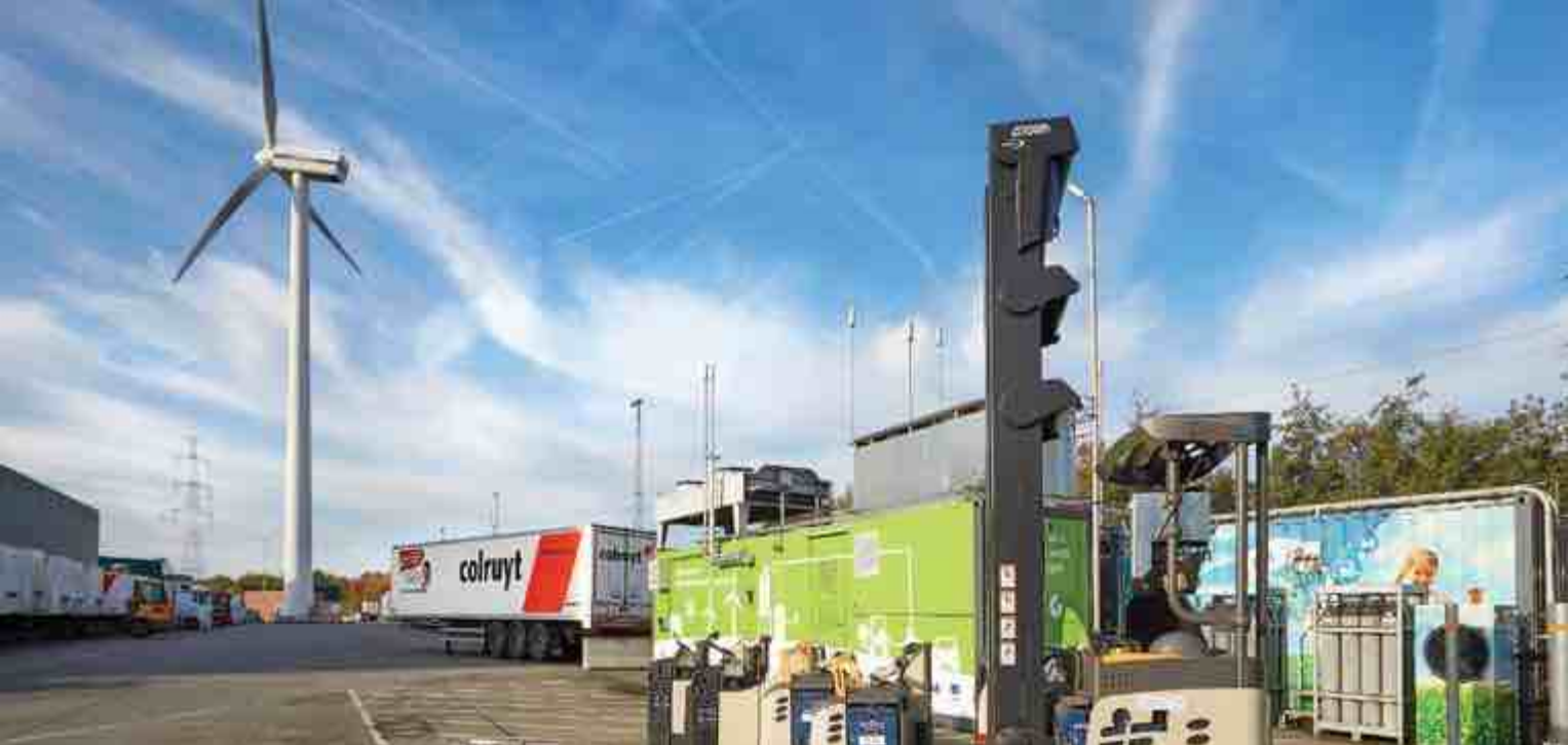
▲ THE CERTIFHY PILOT PLANT COLRUYT GROUP PRODUCES GREEN HYDROGEN ON SITE FOR FORKLIFT FLEETS, HEAVY DUTY VEHICLES AND PASSENGER CARS.
