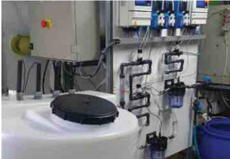
SOLAR PHOTOELECTRO-FENTON PROCESS AT DEMEAUMED DEMONSTRATION SITE (LEITAT, WWW.LEITAT.ORG)
