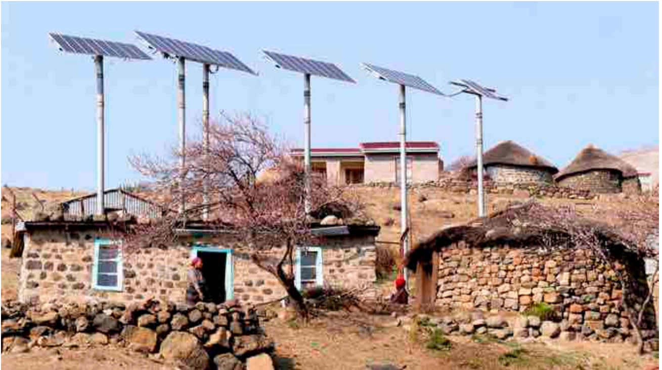
Solar panels in a village, Lesotho.
