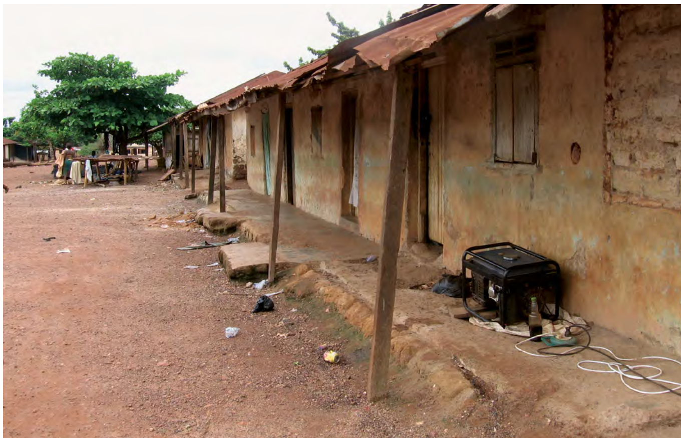
Diesel generator set supplying electricity to the mobile phone charging shop.
